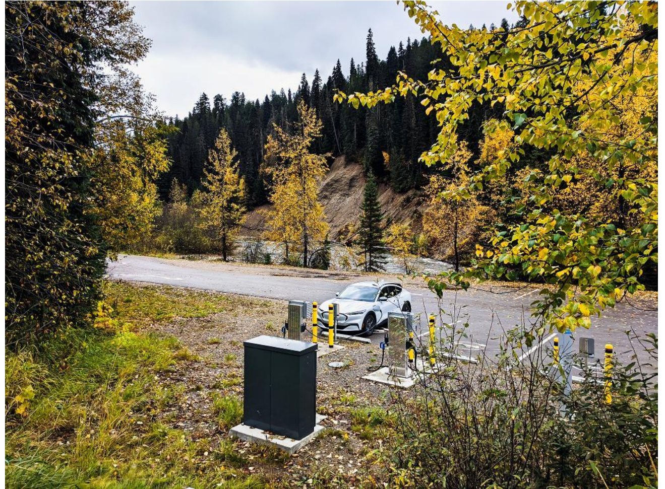
Image: 25 kW charging stations at Slim Creek Rest Area, HWY 16 East
